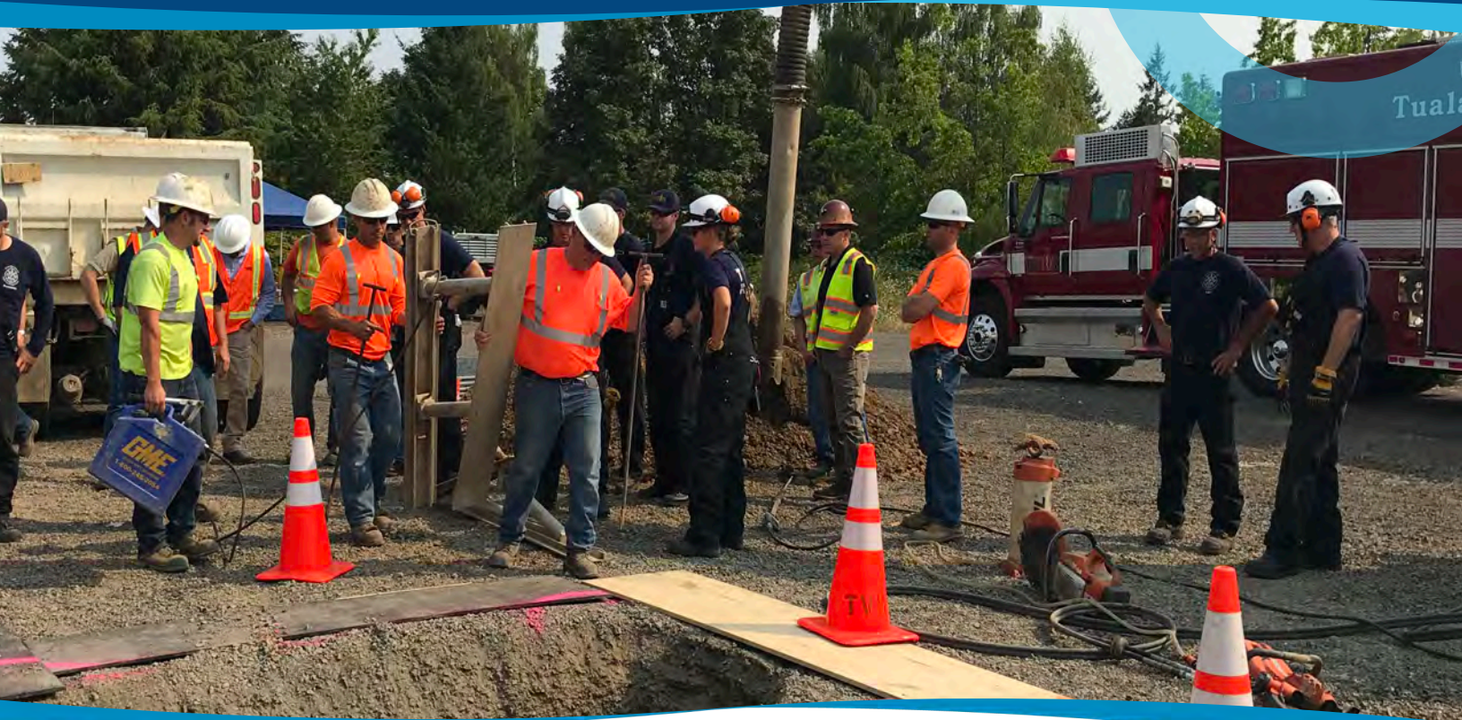
District staff partnered with Tualatin Valley Fire and Rescue firefighters for trench training
