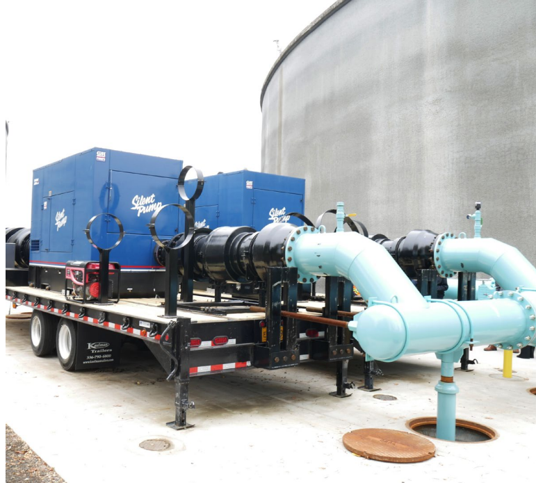
Emergency Interties Emergency Pumping
