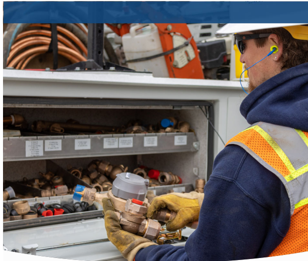
Maintenance and operations of the water system
