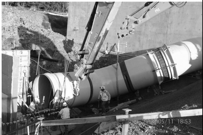
84-inch yard pipe at FWPS
