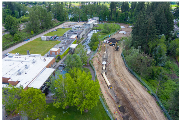
66" pipe in Park
