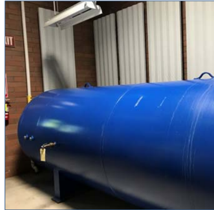
Need Additional Air Receiver Tank
