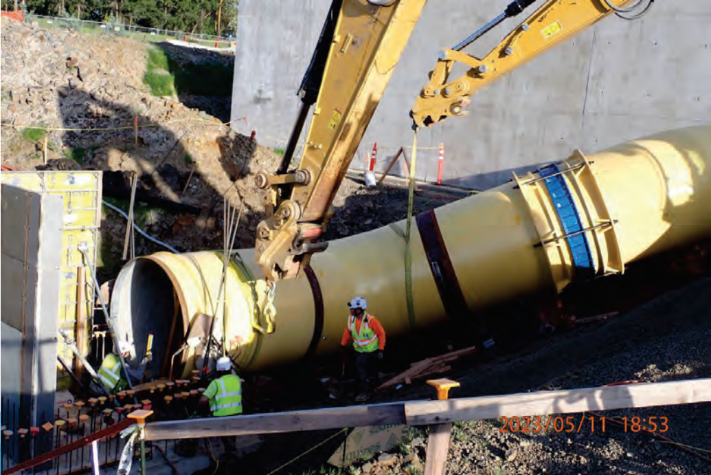
84-inch yard pipe at FWPS
