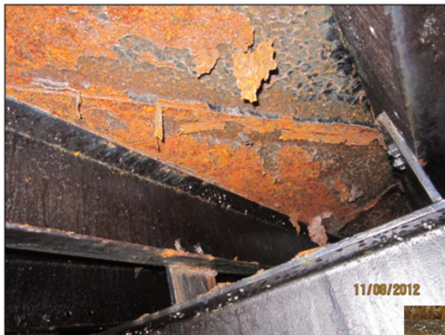
Reservoir Interior Ceiling – Very Poor Condition, Severe Corrosion
