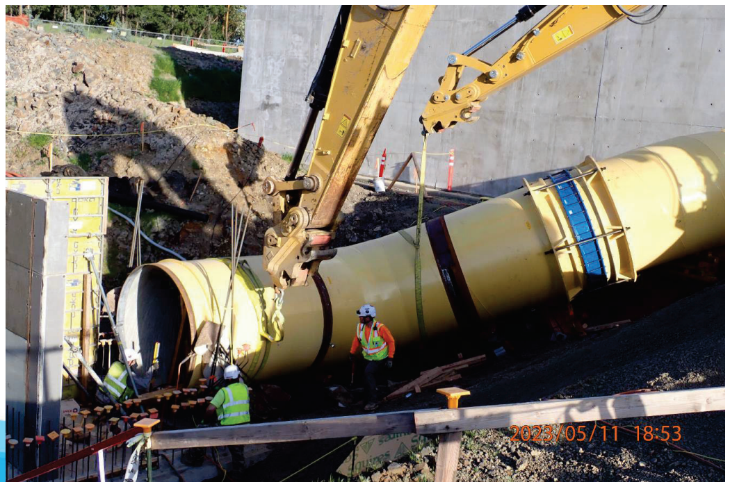
84-inch yard pipe at FWPS
