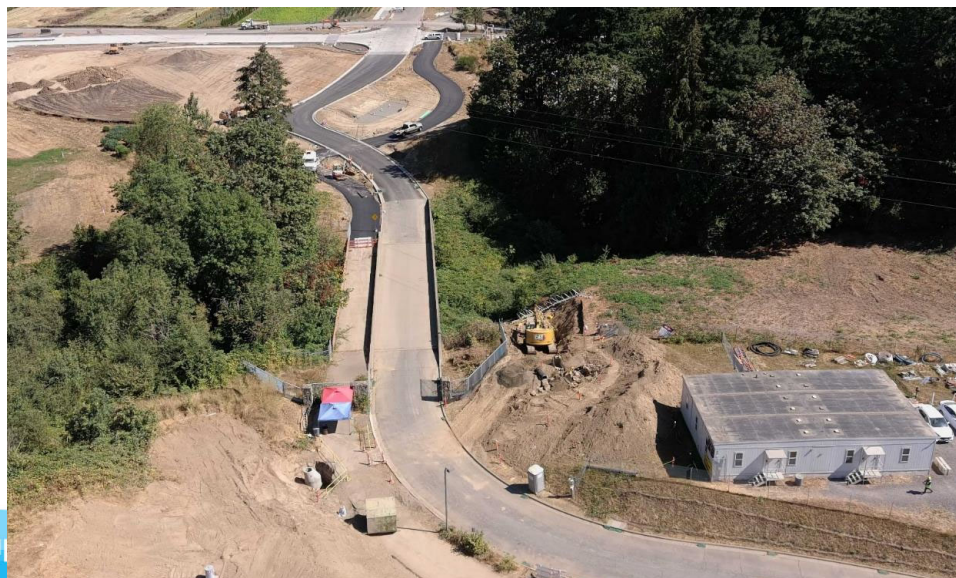
Upper Site Utilities: 18" SD from Upper Site Bioswales to Arrowhead Creek outfall
