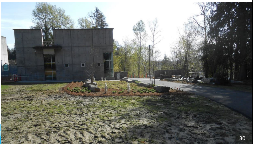
Raw Water Pump Station, Main Overlook, landscaping
