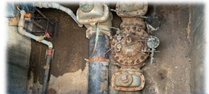
Control Vault at Taylor's Ferry Facility
