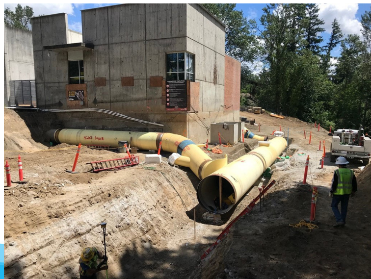
Header piping at Raw Water Pump Station
