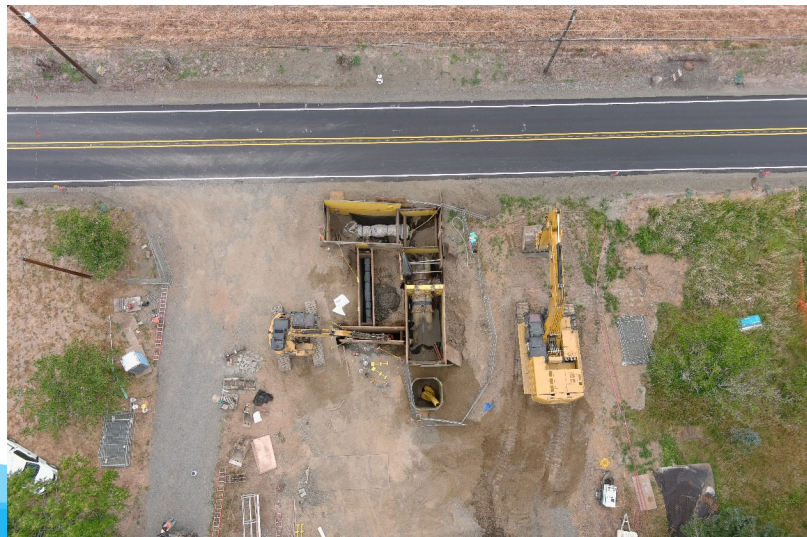
16-inch bypass and 30-inch turnout pipe installation at connection to 66-inch transmission line
