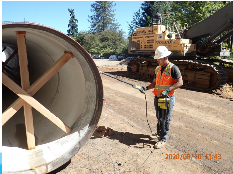
Holiday Testing 66-in Pipe prior to flying in for fit up and installation
