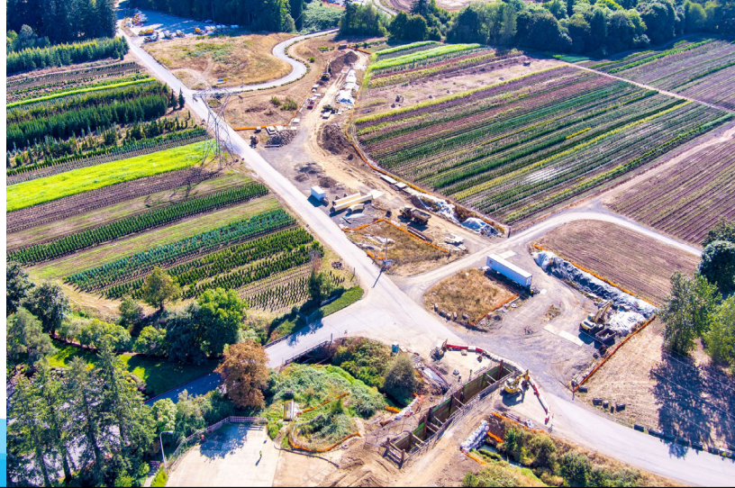
Aerial overview of site, looking SE. Coffee Lake Creek Crossing in fore
